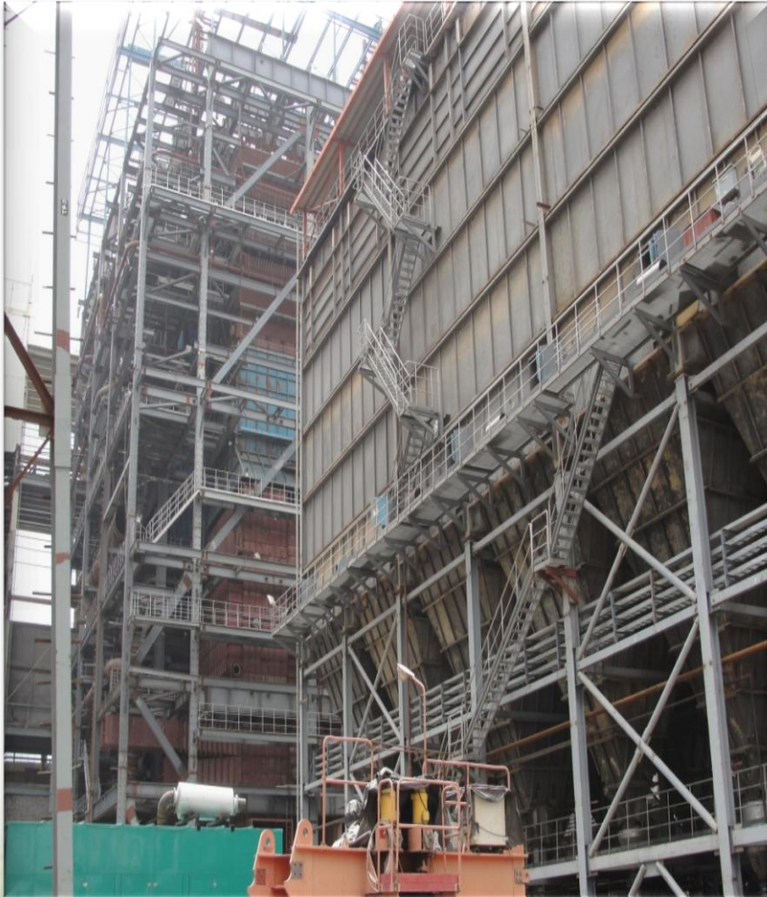
Unit 5 Boiler & ESP
